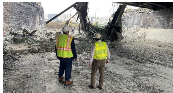
Figure 1. FHWA I-95 Bridge Collapse Inspection (U.S. Federal Highway Administration, 2023).
